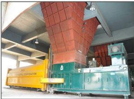
Semi Closed Type Transfer Station with waste compression and Chute system easing waste handling
